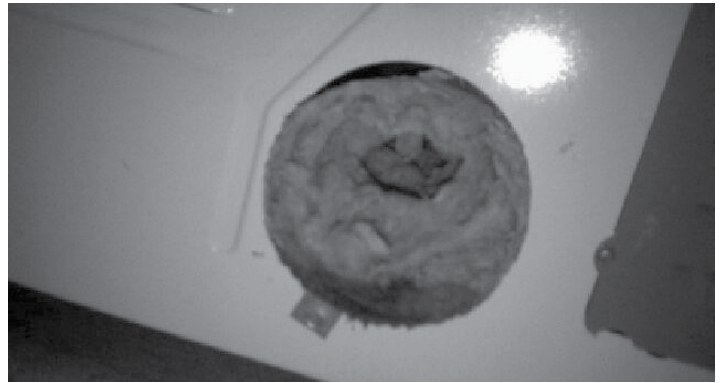
The back port to a dryer that is completely plugged. This is a serious fire hazard.
